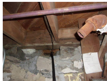
(5) Foundation areas with air leaks (found many like this)
