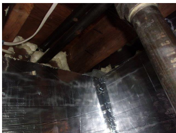
(2) Foundation areas with air leaks (found many like this)
