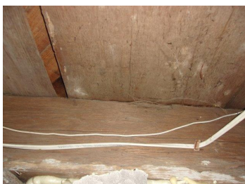
Uninsulated sill beam in the basement
