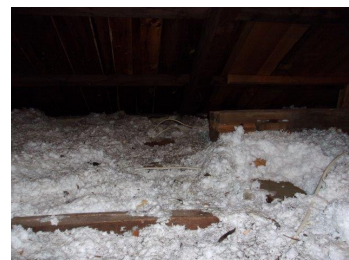
Old insulation in attic area
