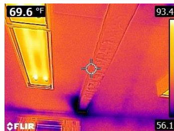
Air leakage in library
