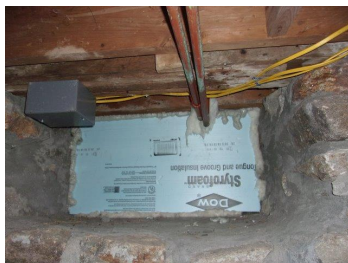
(4) Foundation areas with air leaks (found many like this)
