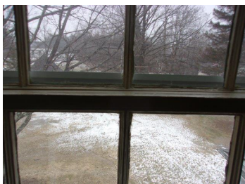
Sash lock is missing
